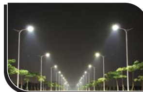
LED Street Lighting
